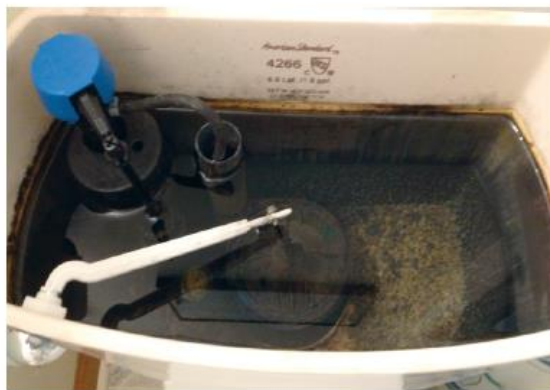
Figure 1. Mn-oxide formation in a toilet tank
